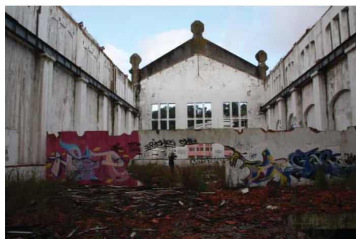
E. Interior Powerplant
