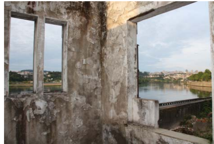
B. Interior pumphouse
