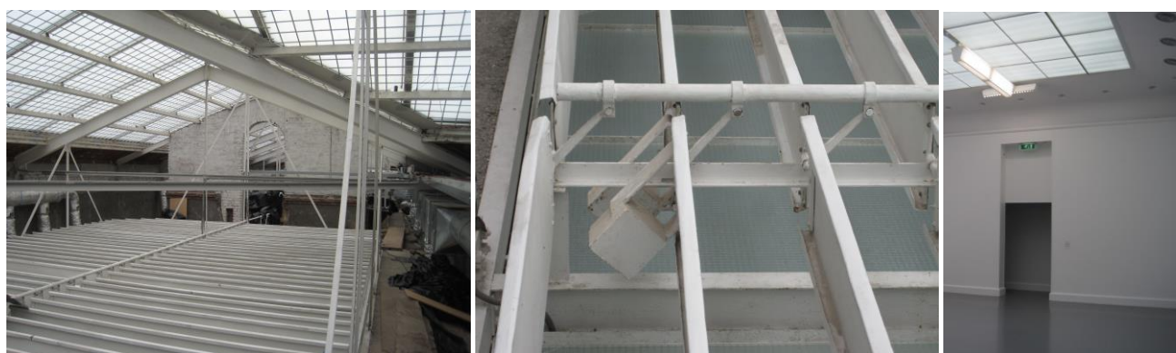
Figure 1.3: Plenum, lamellae detail which can regulate the light transmission into the exhibition rooms, and exhibition room.
