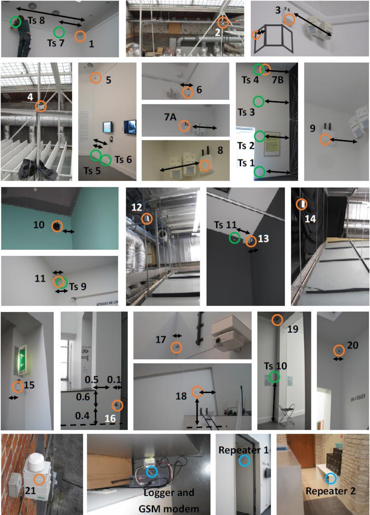
Figure 9.31: Exact locations of the logger, repeaters and sensors. Orange circles represent T/RH sensors, green circles represent T_s sensors.
