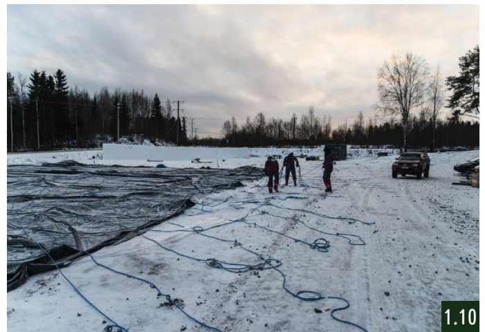
Connecting the rope net to all anchor points to make ready for inflation
