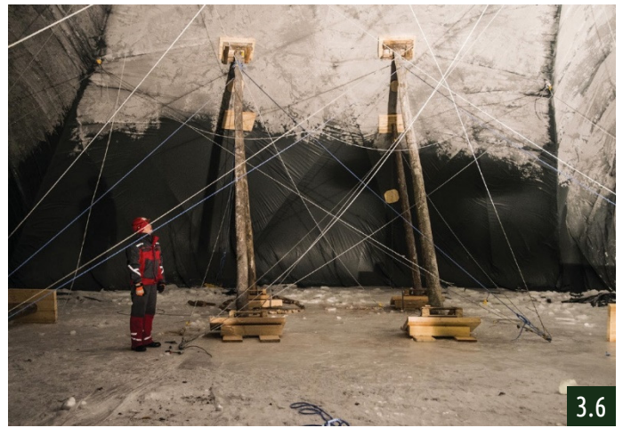
3.6 Positioned columns inside the inflatable to support the bottom part of the bridge
