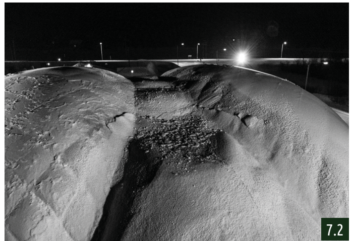
The monitoring system was warning us that the top part of the Bridge was slowly coming down. We were able to close the bridge, but the structural shape did not form a proper arch, which made the Bridge weak
