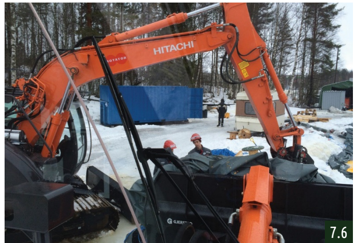
Cleaning the building site to let the scheduled opening festival go on
