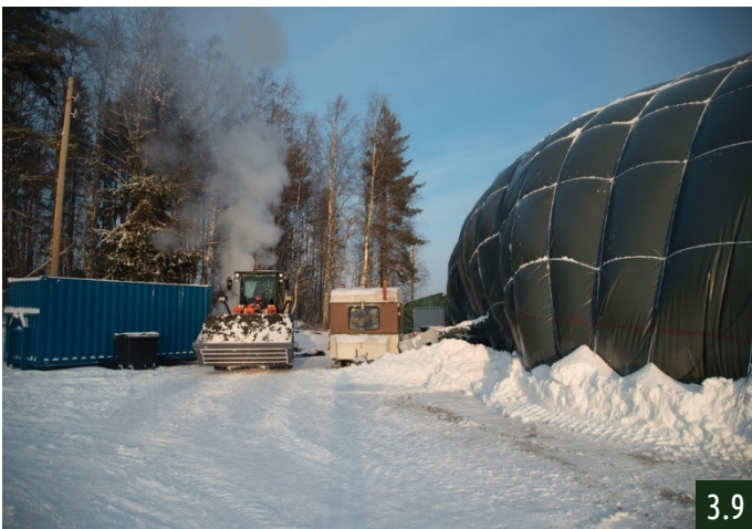
3.9 The side parts of the inflatable are made air tight with snow on the outside, and ice on the inside. The caravan is the control room for measuring and monitoring the inflatable.
