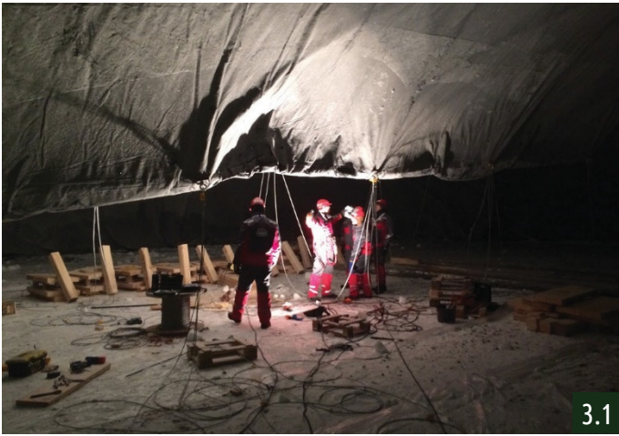
3.1 Connecting steel cables inside the inflatable, to make it stable against wind gusts
