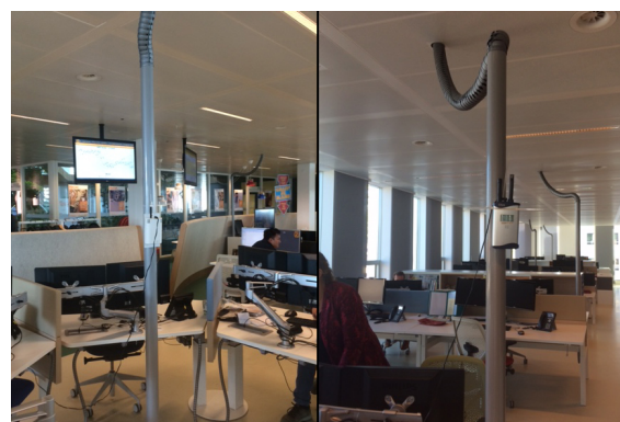
Fig. b1.1: Data loggers on the second floor. Left: room 2.1, Right: room 2.2.
