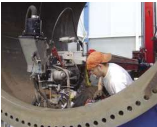
Figure 4.20 A technician prepares equipment to weld a flange to a tower part (Lincoln Electric, 2010)
