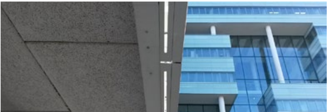
Figure 1.1: Application of WWCBs at the Flux building on the campus of Eindhoven University of Technology.
