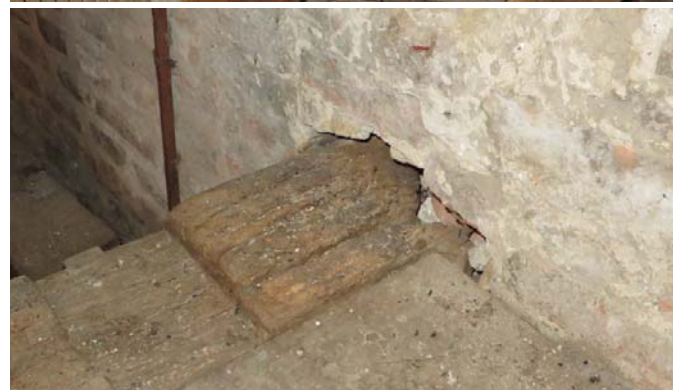
Figure 4.2 Wooden beam end (bottom) as part of the internal construction (top) of a church in Beusichem. The end desintegrated and isn't connected to the wall anymore.
