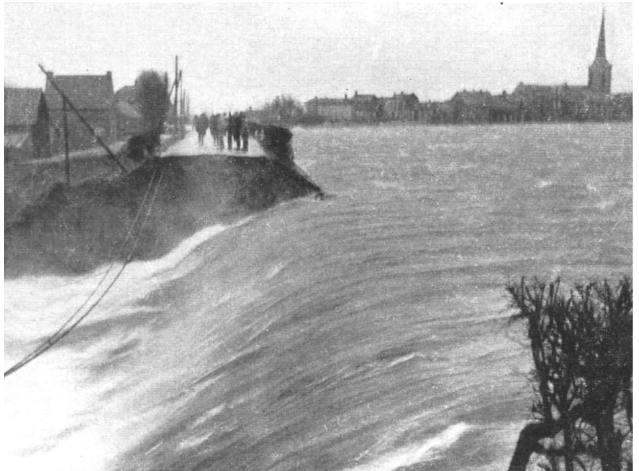
Fig. 1: Breach at Ouderkerk aan de IJssel, upstream along the tidal reach of the river Hollandse IJssel, at the time of tidal low water (from Van Veen 1962).
