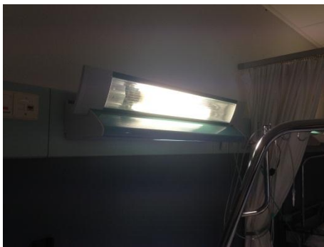
Rotating indirect lighting
