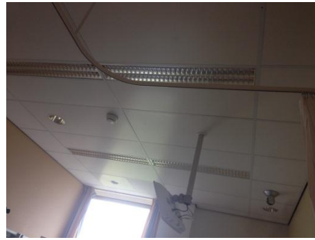
Lighting situation, dimmed luminaires
