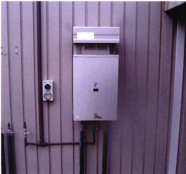
Figure 24. Gas water heater placed in metal box in the sun
