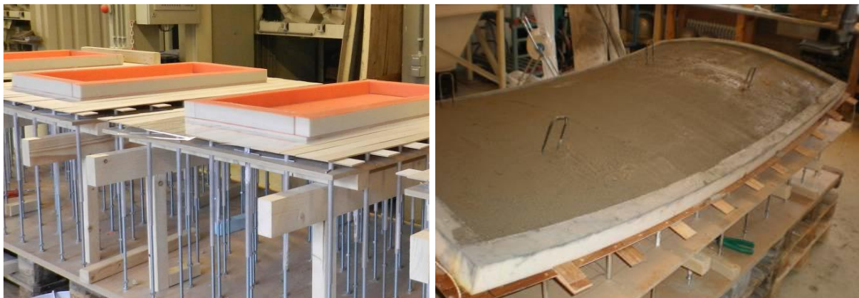
Figure 25a: The principle of the moulding technique (Schipper, Grünewald, Eigenraam, Raghunath, & Kok, 2014) & Figure 25b: Poured concrete on the flexible mould (Janssen, 2011)
