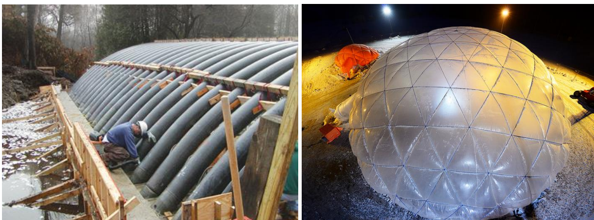
Figure 20a: Kenway Bridge (Kenway Corporation, 2014) & Figure 20b: Pykretedome of the Eindhoven University of Technology (Van Overbeeke, 2014)
