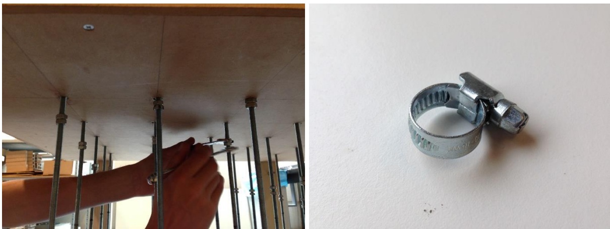
Figure 93a: Setting the height by the use of nuts & Figure 93b: Hose clamp
