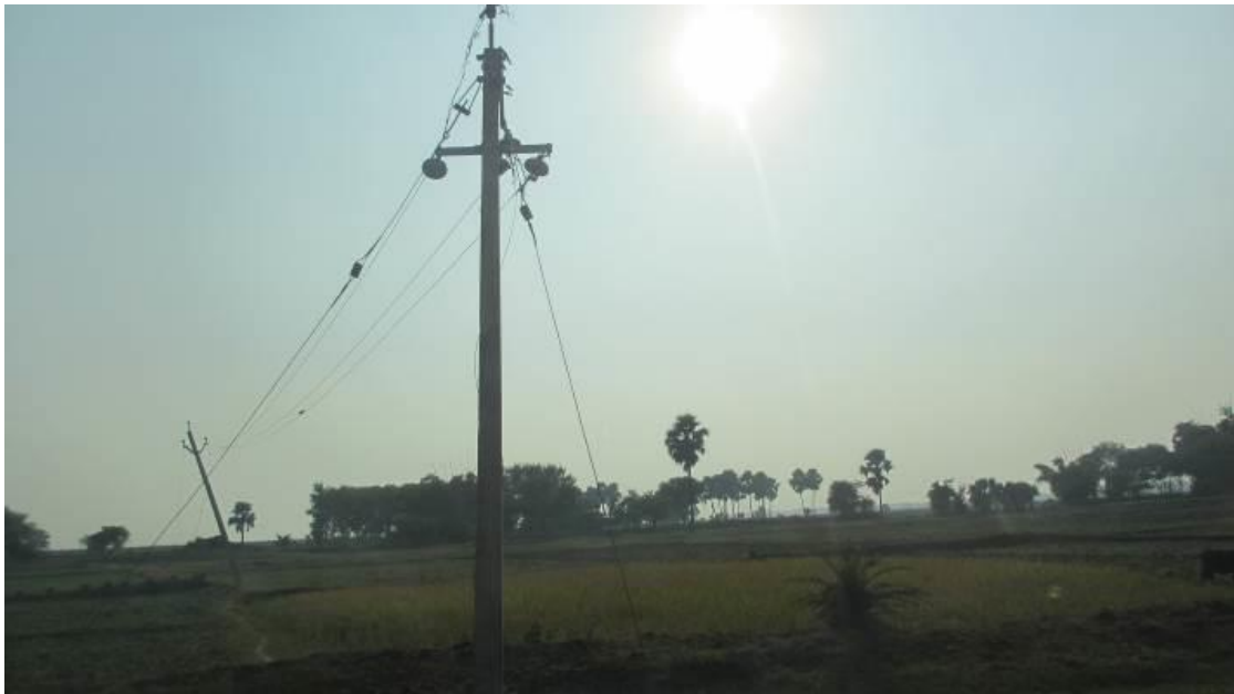
Figure 3-1 Electricity poles with broken wires. The wires are stolen and to sell the cooper.
