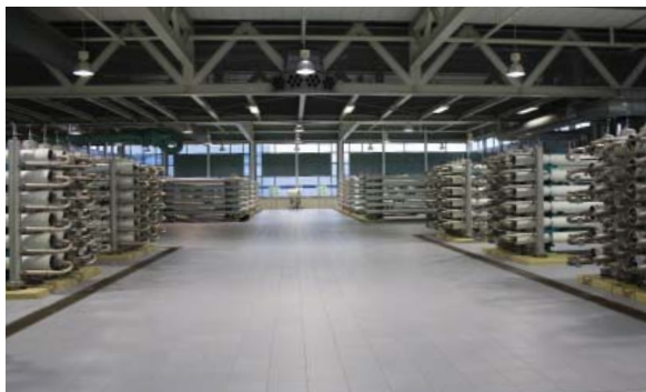
membrane filtration (plant in Heemskerk)
