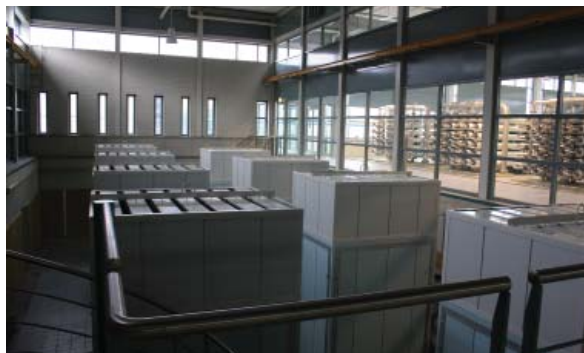
pumps (plant in Heemskerk)
