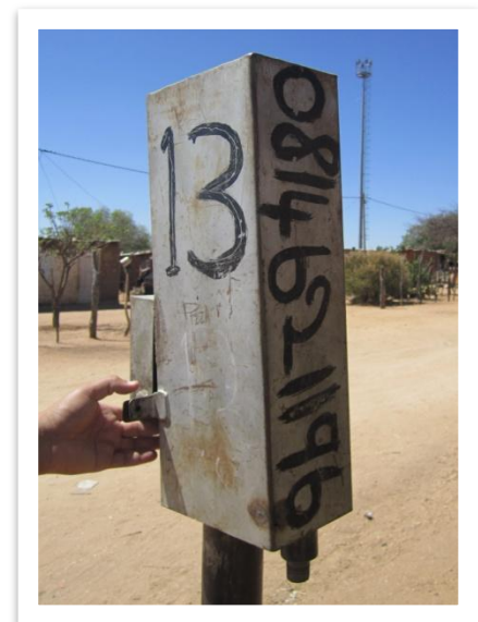
Figure 14: A standpipe (no. 13) in the informal settlements, fitted with a prepaid meter (not visible) and the phone number of one of the municipal technicians written on the side.
