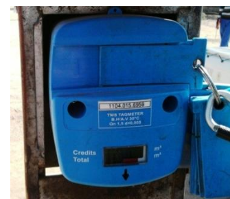
Figure 5: Prepaid water meter with tag inserted.
