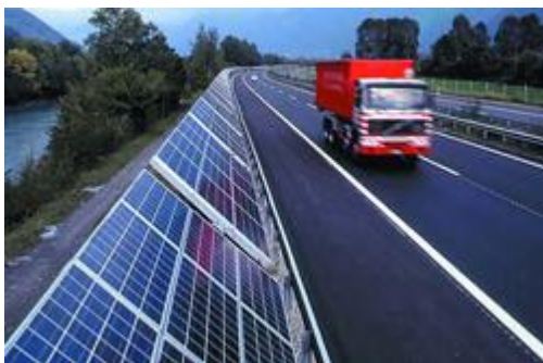
Figure 16: PV system near A13, Switzerland.
