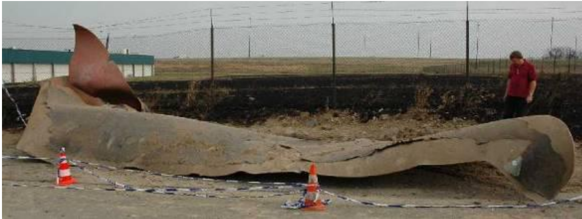
Photo 7: The missing piece of pipe (Belgium Min. Econ. Aff.)
