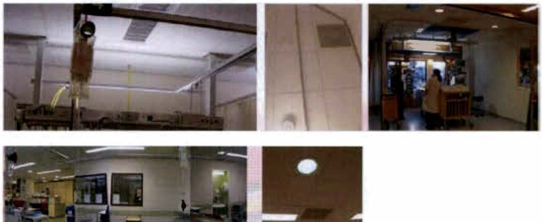
Figure: Ventilation devices of respectively THIC, ICB, and CHIC
