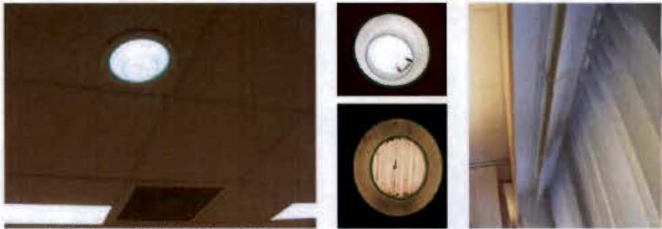
Figure: Existing artificial lighting at ICB
