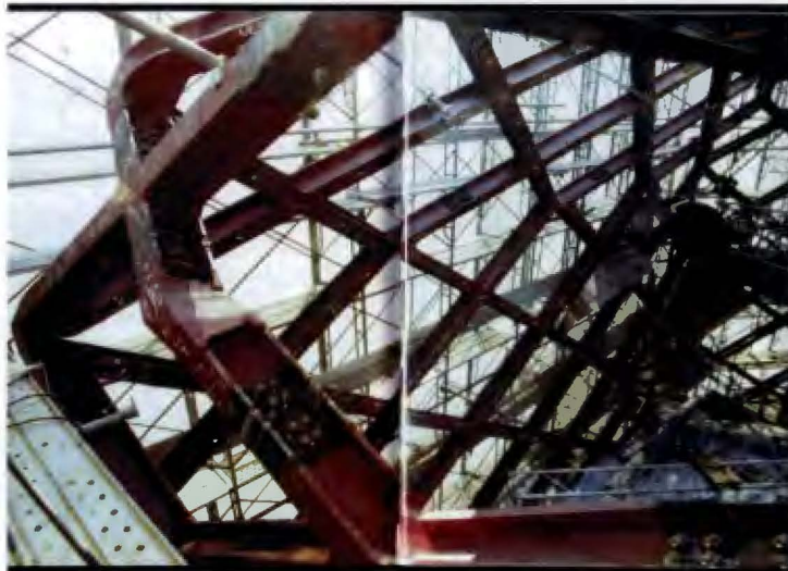
Steel frame from Prada store; Architects Herzog and the Meuron (source: scan from book Prada Aoyama Tokyo )
