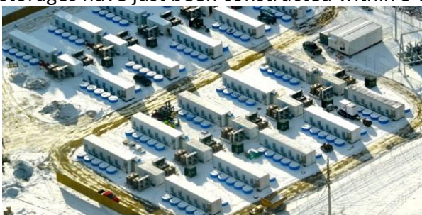
Figure 13: Flywheel frequency regulation energy storage system (Stephentown, New York, USA)
