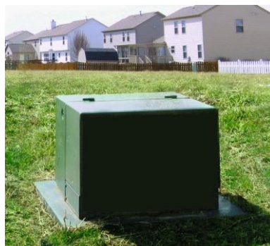
Figure 18: A 25 kWh Community energy storage installed in Ohio (USA)
