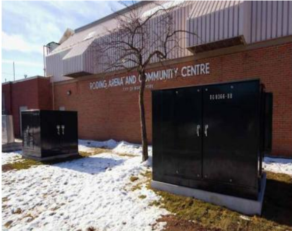
Figure 16: Community energy storage
