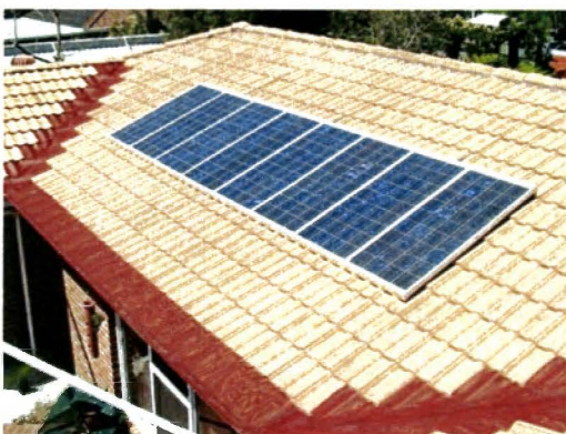
Figure 46: Example of a roof top area covered by 8 m 2 crystalline PV arrays [45]
