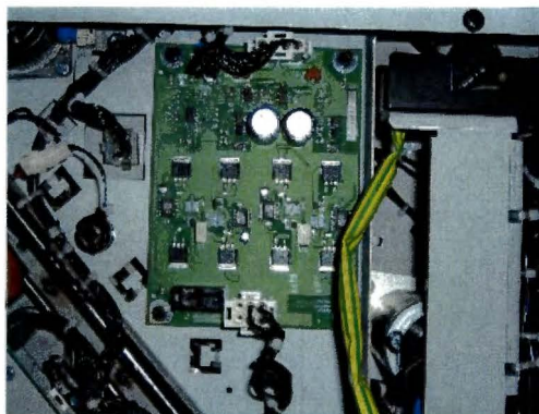
Figure 8.219d Power electronics board
