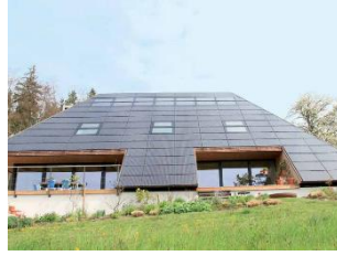
Figure 34: BIPV full roof (2)
