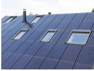
Figure 33: BIPV full roof (1)
