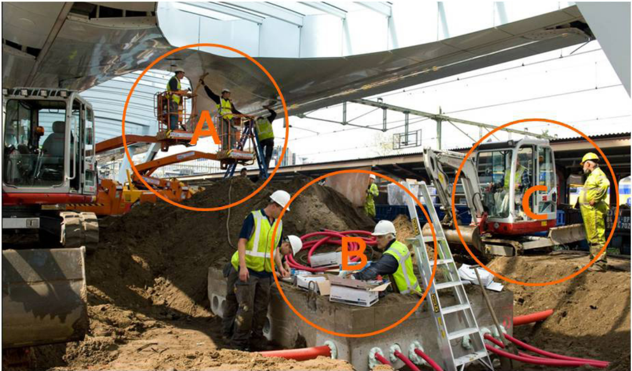
Figure 9.6 Typical scene showing the difficulties of operating in a giant sand-box with less work space. Co-maker (A) Sorba is finishing the ceiling, co-maker (B) Spie and co-maker (C) Dura Vermeer are working in the ground respectively on installations and the bedplate.
