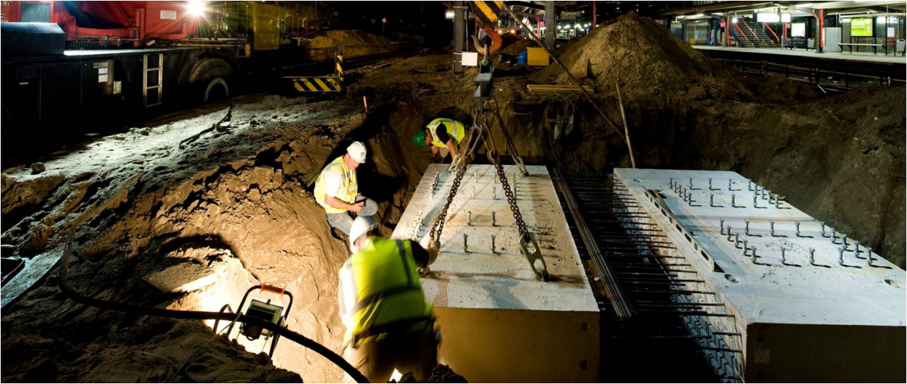
Figure 7.22 Much work is performed during night and weekend hours, like positioning the prefab foundation elements.
