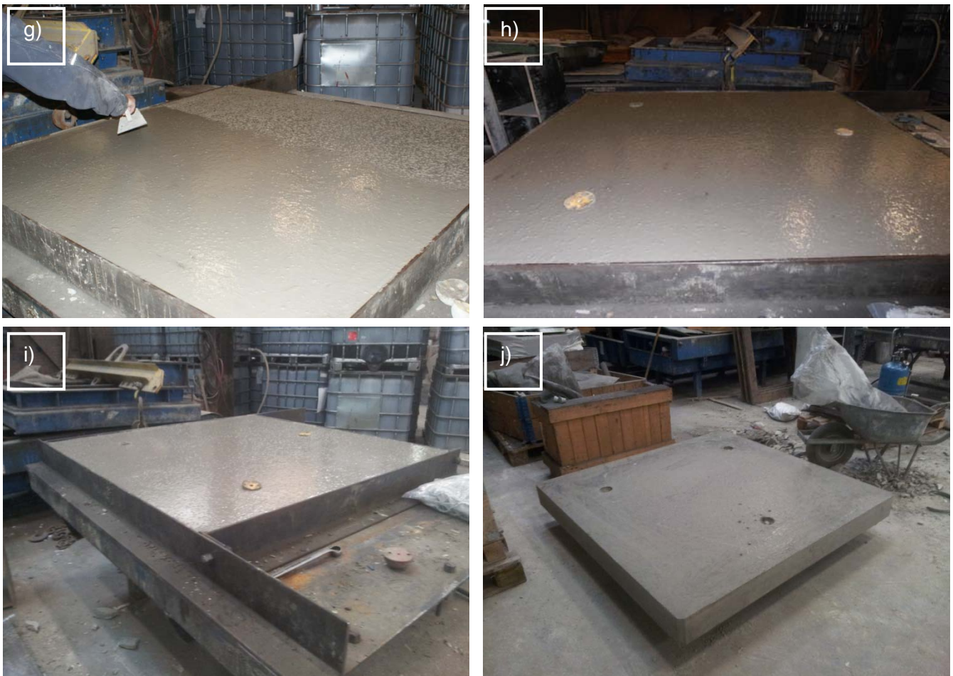
Figure 6-11; e-f) de-airing SCC, the entrapped air comes out of the concrete and forms a top layer of bubbles, g) wiping the air bubbles of the concrete to get smooth surface, h-i) the casted element must stand for 16 hour, before demolding it, k) the element after 16 hours of hardening after demolding
