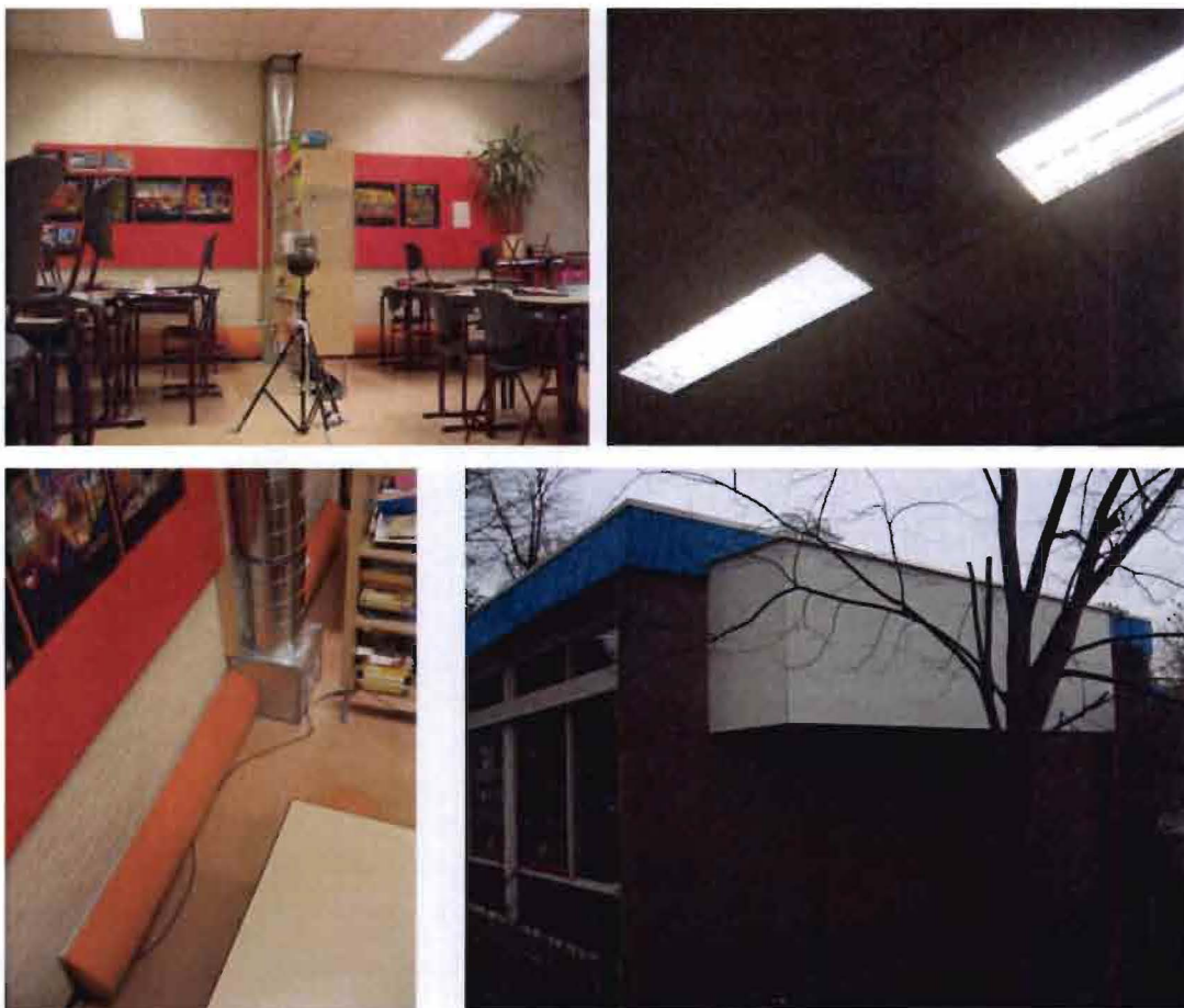
Figure 3.3 Upper left: The supply duct system and the measuring tripod
