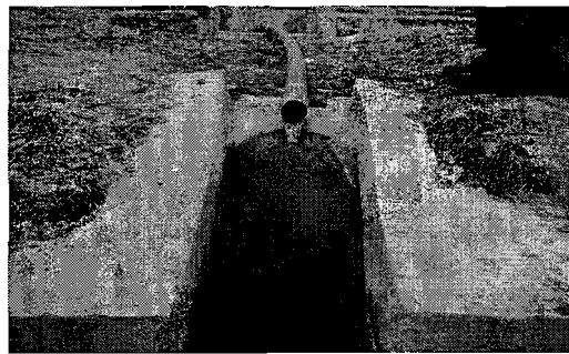
Figure 25 the clean effluent runs to the land
