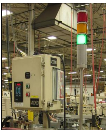
Figure 2.3. Machine stack light.
