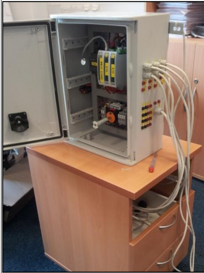
Figure 3.10. The PLC with its components, such as a power supply and input - and output - connections.
