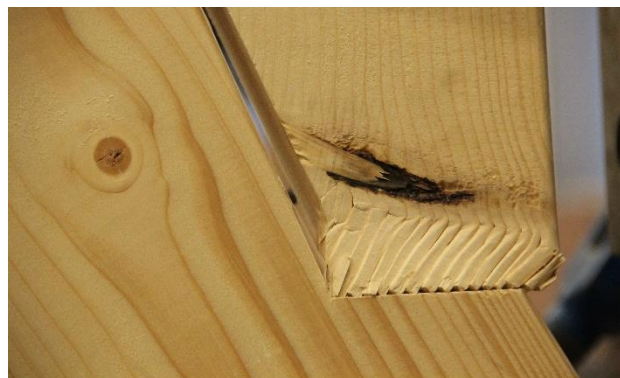
Figure 47: Butting failure of the diagonal element due to an imperfection causing a different growth-ring orientation.
