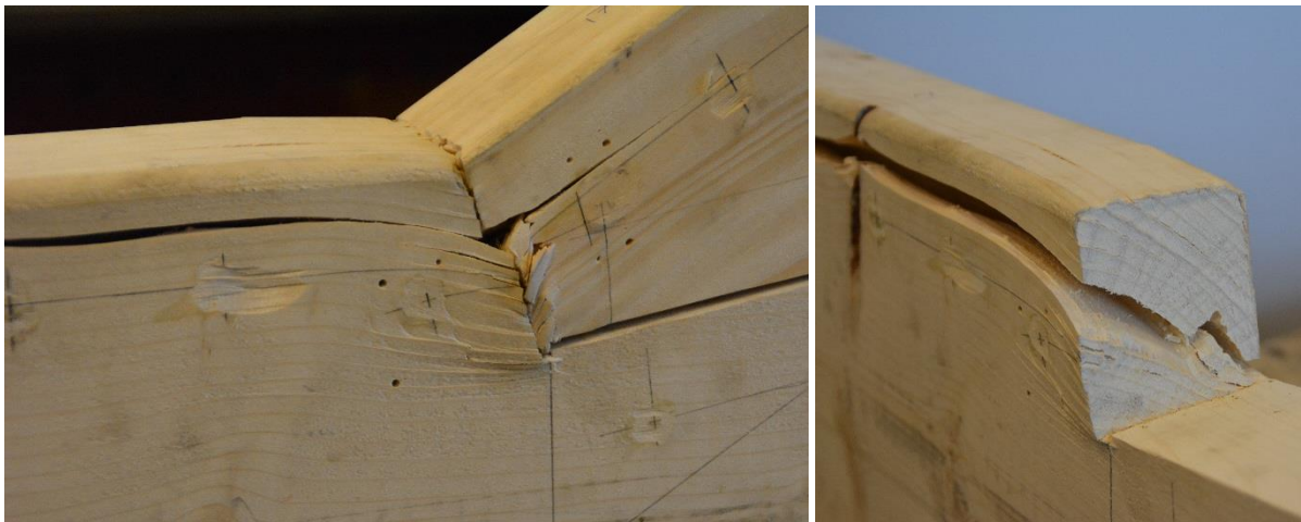
Figure 43: Shear failure after butting of the front notch
