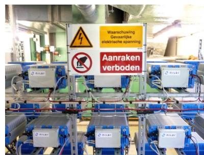
Fig. 6.4.1: BESS safety signs placed on rack and at room entrance
