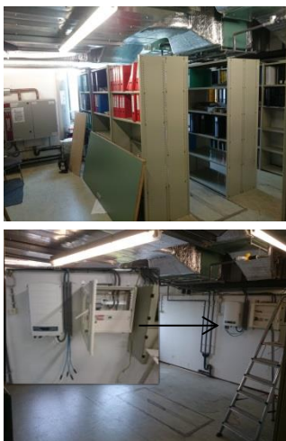
Fig. F.2.4: Installation room: before, and after new PV-inverter (12yrs warranty) and electrical distribution box (LK 2020) for connection of PV-system (32A MCB) and ESS(40A MCB)
