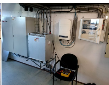
Fig. 6.1.3: Accuracy measurements KEB-cabinet (III)
