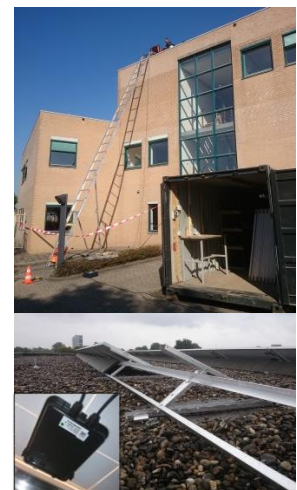
F.2.7: Temporary storage and vertical transportation. Panel construction, with maximum weight (~300 tiles of 4.5x30x30cm) for optimal safety against high wind gusts. Picture below show the panel integrated optimizer (25yrs warranty).
