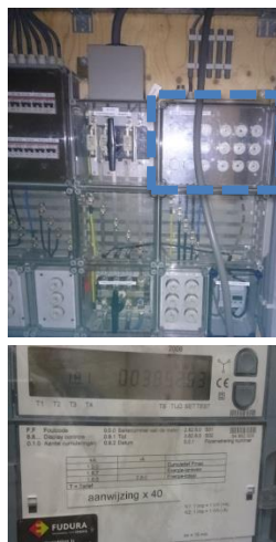
Fig. F.2.5: Replacement of existing 6 x25A fuses to 4 x 63 to connect PV+ESS distribution box. Empty group for Electric Car charger. Register installation at Utility (Enexis), new contract: 53kW consumption and 150kW production (transportation only charged for consumption)
