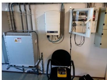
Fig. 6.1.1: Accuracy measurements for central BESS energy meter (II)
