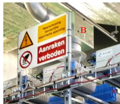
Fig. 5.4.2: Safety-signs (A) & Ventilation outlet (B). Ventilation capacity setting (unverified): 500m 3 , installed after cooling block north-east ventilation group
