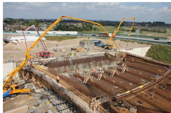
Figure A.0.2. Fixation of the reinforcement steel, the main task of the subcontractor
