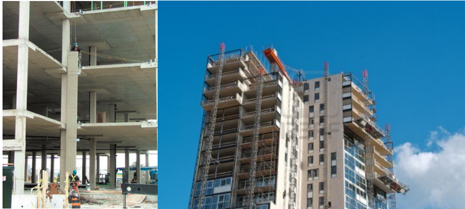
Figure 6.7 Building mass of a concrete structure can be used as a heat buffer.
