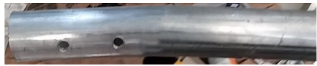
Figure 104: Plastic deformation of compression element near connection
