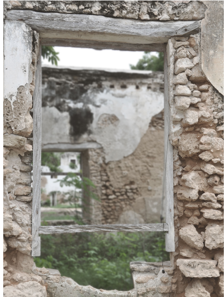
Image 6 - Severely degraded traditional opening in a coral limestone wall
