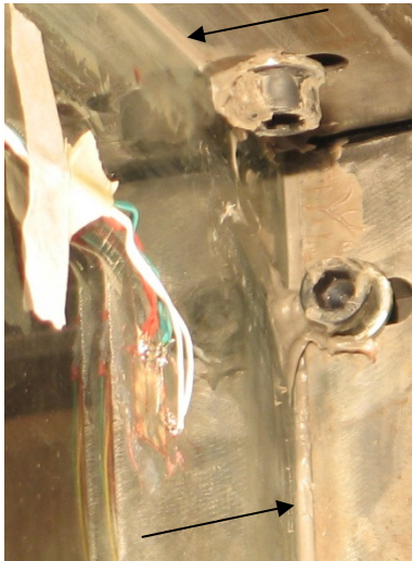
Figure 4.24 undamaged adhesive bonded joint. (HSG 1 before testing)
