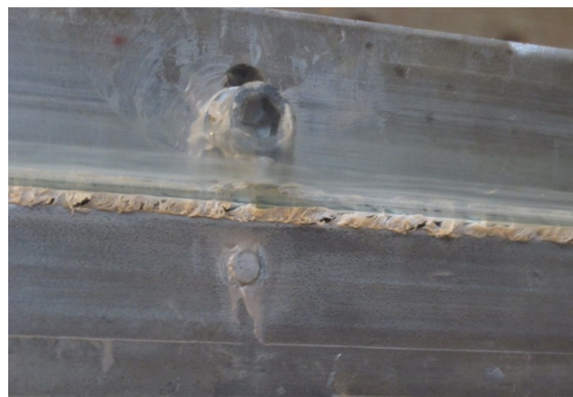
Figure 4.27 Close up failed adhesive bonded joint. (HSG 1 after glass pane failure)
