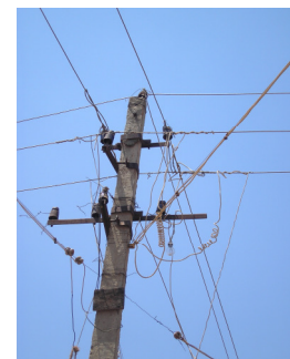
Fig. 5.3: Illegal connections to the grid power
