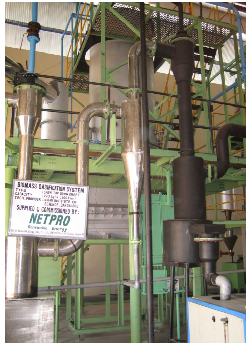
Fig. 6.4: The 200 kWe BERI biomass gasifier, built by Netpro
