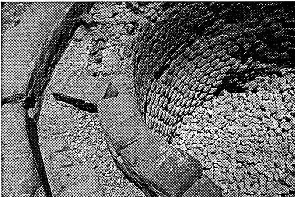
Kiln wall (Mvumi) The brick lining has deteriorated seriously. Burnt quicklime lumps at the bottom of the kiln.
