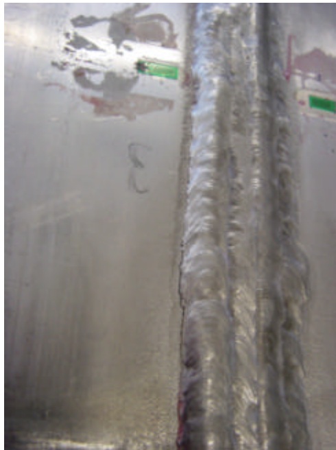
Figure 4: close up of the cracked welded joint
