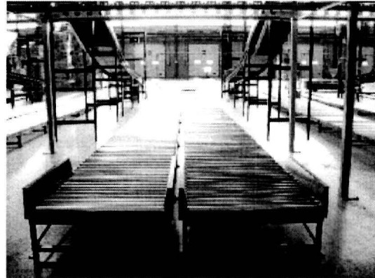
Photograph 4: Lanes (roller conveyors), one on each side of the chute (sorter under construction)
