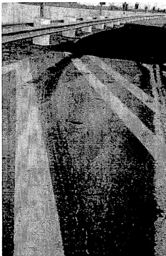
Figure 15: cracked asphalt and patched area, source: AFRICON
