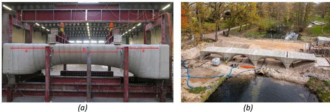
Figure 1-2: The setup of the structural mock-up test of Nijmegen 3DCP bridge(a) and the assembly of final bridge on location(b), as described in [12].
