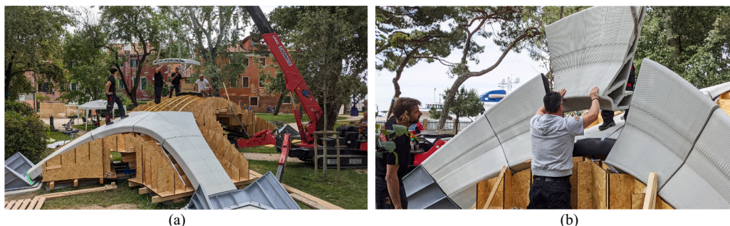
Fig. 7. a, b. Assembly of the Striatum Bridge. The elements were found to have sufficiently accurate dimensions to be placed without additional adjustments.
