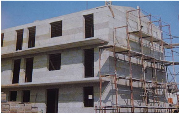
Figure 5 - Permanent Shuttering Boards
