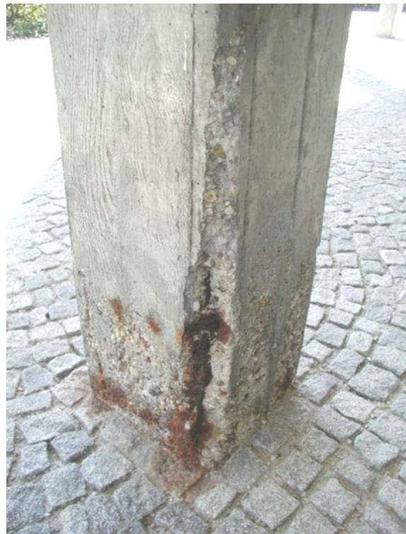
Figure 1: Mechanically loaded concrete column, affected by chloride in de-icing salts which has induced corrosion of rebar and freeze-thaw scaling, photo Gehlen
