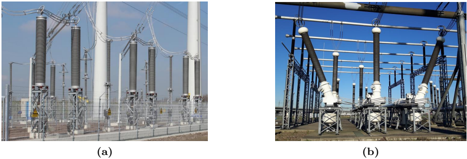
Figure 5.7: (a) Representation of the transition point configuration; (b) configuration of one circuit at substation BWK.
