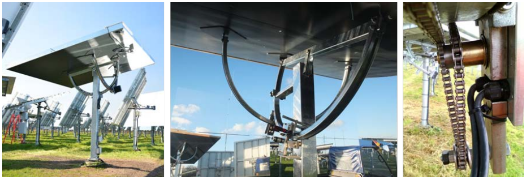
Fig. 14: DLR 9m 2 rim drive heliostat with chain gear avoiding fluctuating tension of the chain caused by the polygon effect
