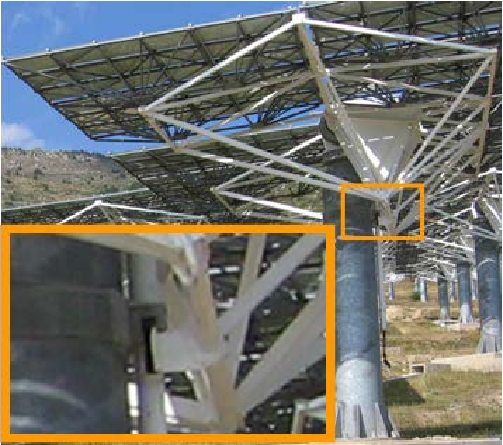
Fig. 10: Locking of elevation drive during stow and framework facets, seen at Themis solar power plant heliostats
