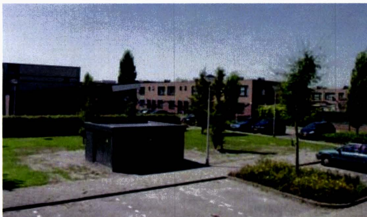
Figure 1.2 Photo of the Smart Storage Unit (SSU), as it is installed in the field at Etten-Leur.
