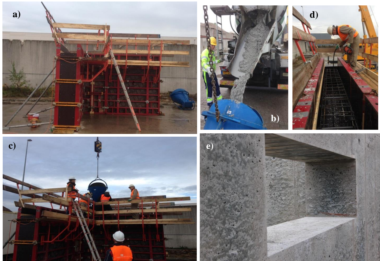
Figure 5. Ultra-lightweight concrete test wall production: a) wall formwork, b) and c) concrete transportation and casting, d) compaction with a needle vibrator and e) demolded concrete wall with a window opening. Photo e) by Dolph Cantrijn.
