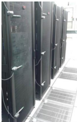
Fig. 4 Photo of demonstration DC
