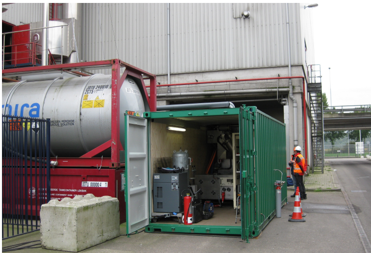
Figure 2.2: Pulsed corona pilot container at a domestic waste handling facility.
