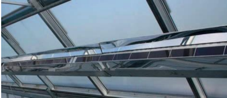
Figure 2.17 A prototype of CPVT installed in DaglichtKas (Zwart & Noort 2012)
